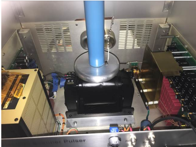
Figure 3. Layout of the HVP components inside the chassis.
